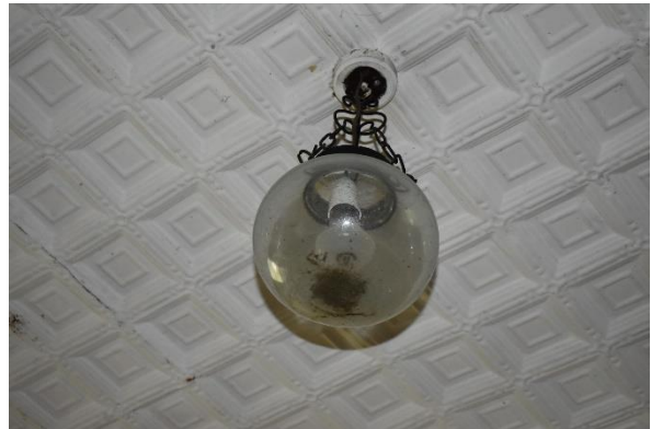
Figure 32. Detail view of the pressed metal ceiling and potentially an original light fixture.
