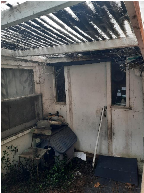
Figure 23. View of eastern side entry into 1956 'maid's quarter' extension. Source: Yarra Ranges Council.
